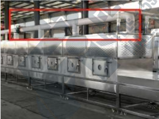
Heat & Moisture Removal System
